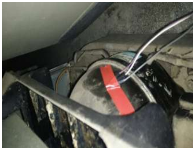
Fig. 18. Measuring and monitoring temperature of compressor unit
