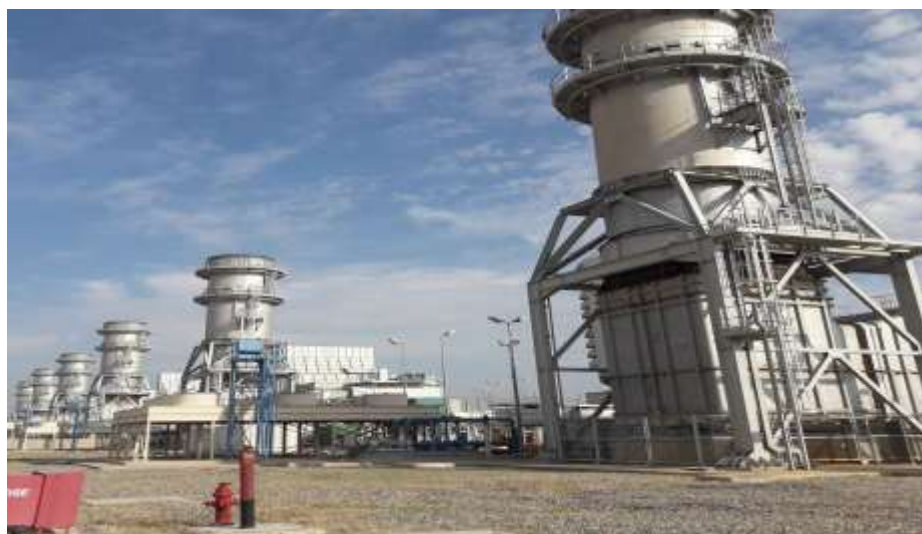
Figure 3. Qayyarah gas power station[14]
