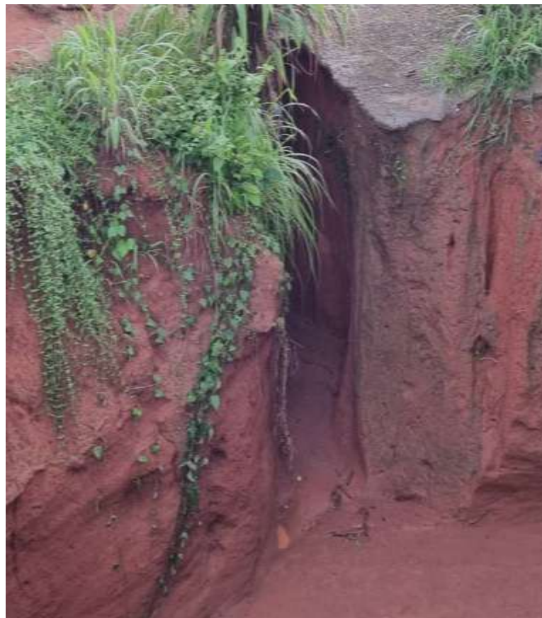
Figure 5: Pictorial evidence of a lack of drainage system in Ijebu Ode, Ogun State
