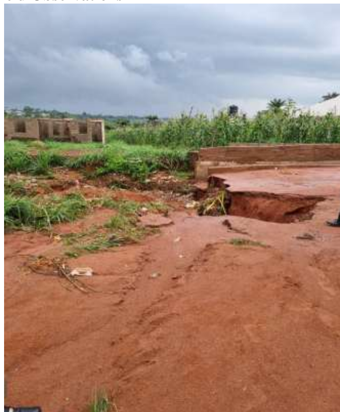
Figure 2: Field observation of collapse drainage system at the study area with evidence of run-off water at Ado-ota Road
