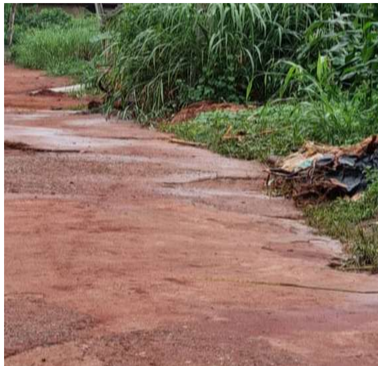
Figure 4: Road destroyed by flood due to lack of standard drainage, creating difficulties for community motorists and Business operations commuters at Abeokuta North.
