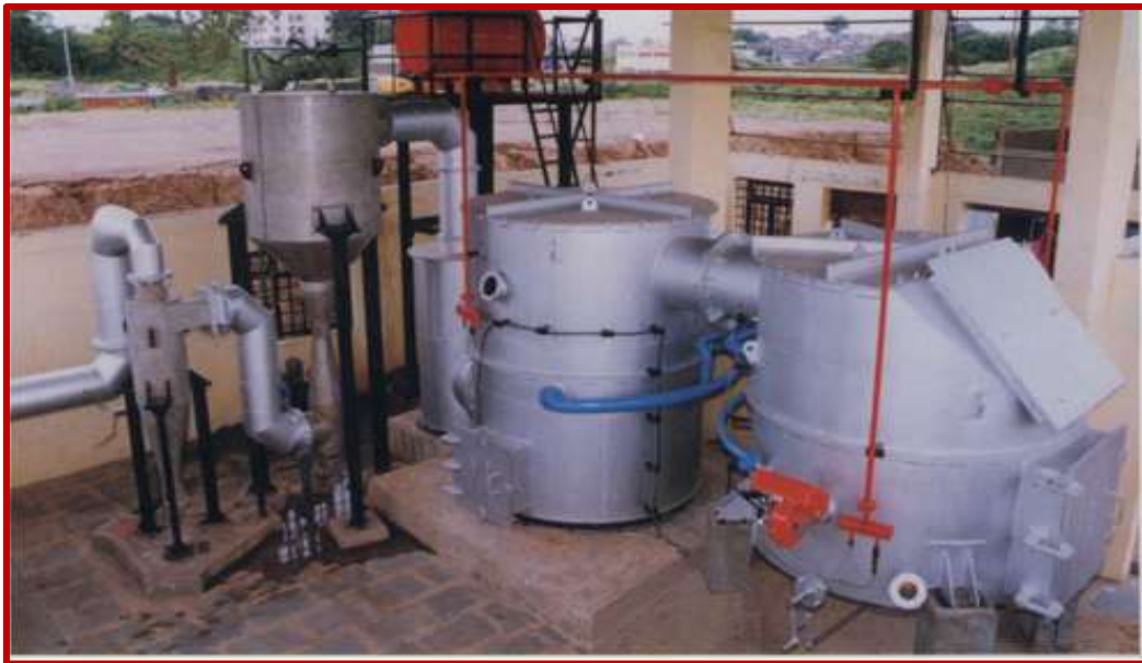
Fig. 7 Flue Gas Treatment at ((Water Grace Products), Nashik
