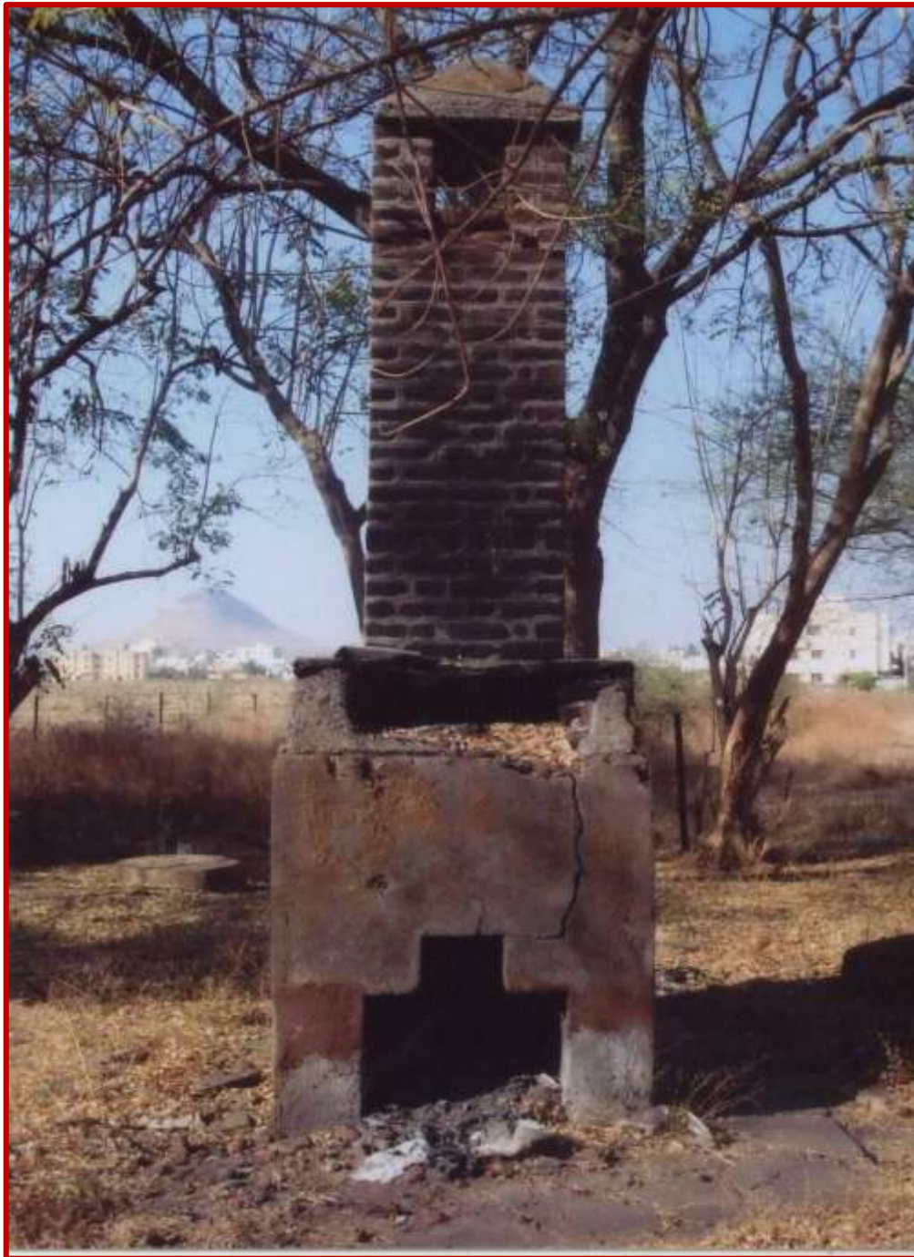
Fig.4 Small Incineration Plant at Maharashtra T.B. Sanitorium
